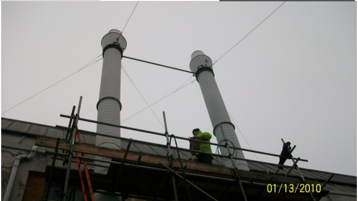
Each of the stacks are identical with common temporary platform access shown.
