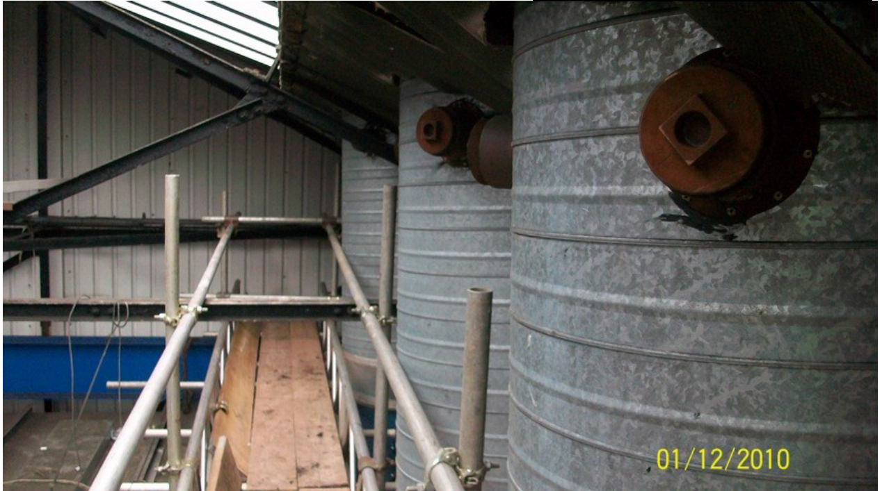
Each of the stacks are identical in dimensions and accessed from a common temporary platform - shown
