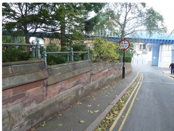
Ornamental railings missing from the west boundary wall.
