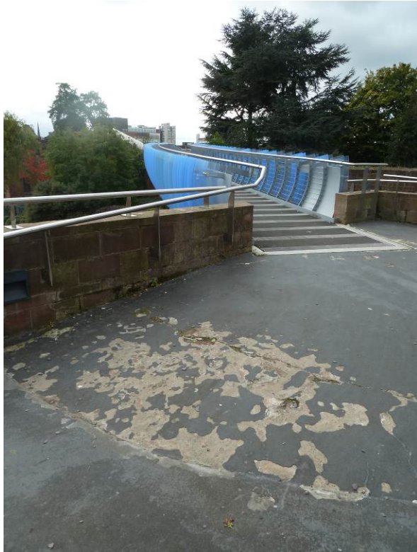
Area of repair needed on viewing platform surface
