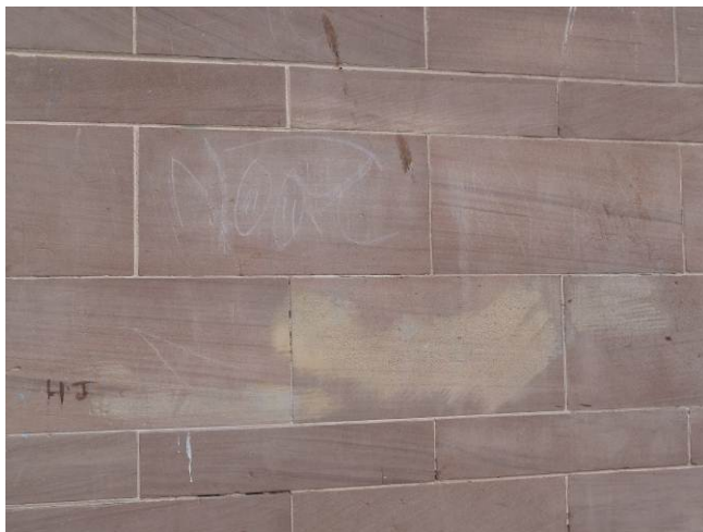
Graffiti on sandstone wall
