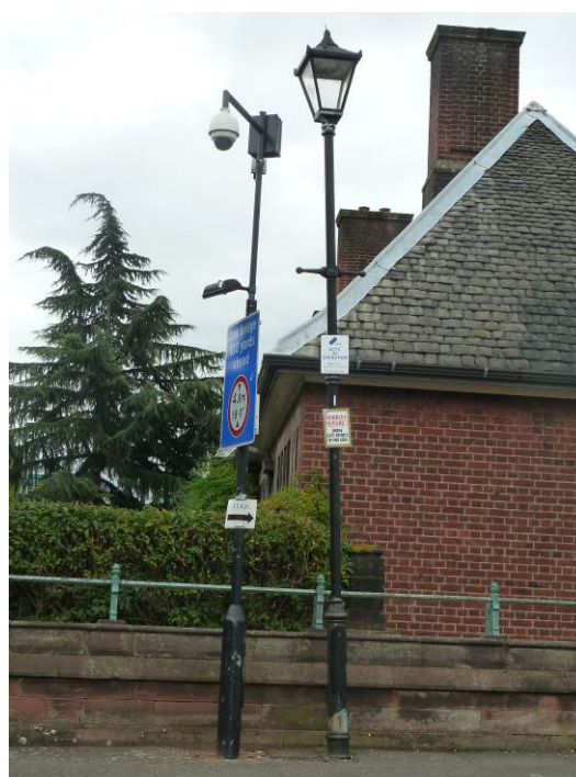
Lamp post and CCTV post located too close to each other with additional signage added to them, which creates a cluttered view
