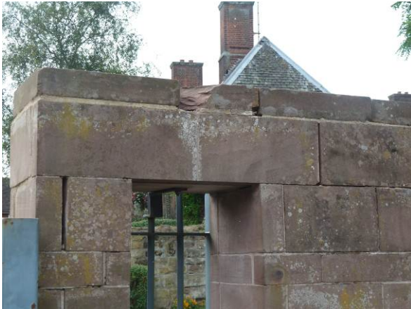
Damage to sandstone wall
