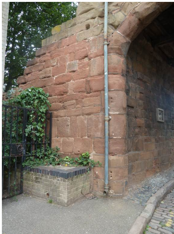
Brick structure built against up against Cook Street Gate from materials that do not compliment the historic building
