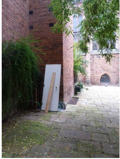
Rubbish left outside buildings in Castle Yard
