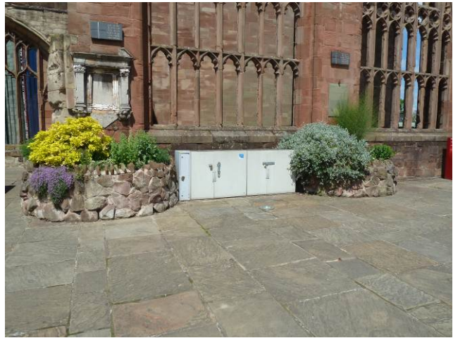
Intrusive cabinets using inappropriate materials within the Cathedral ruins
