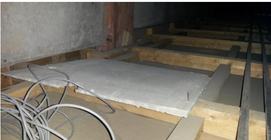
Asbestos firebreak in ceiling void of a school
