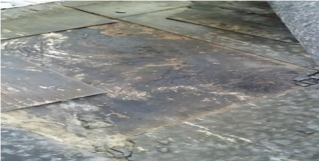
Floor tile adhesive (Bitumen) containing asbestos
