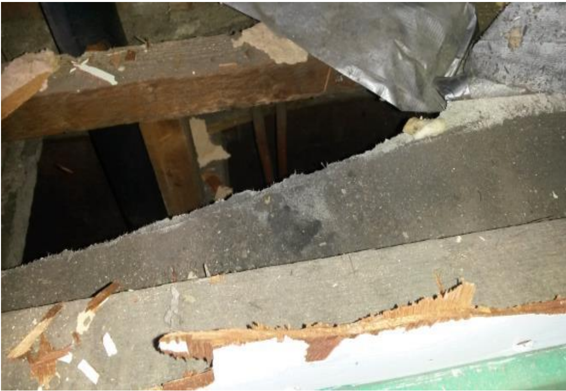
Damaged asbestos panelling – AIB base board to riser, historic damage
