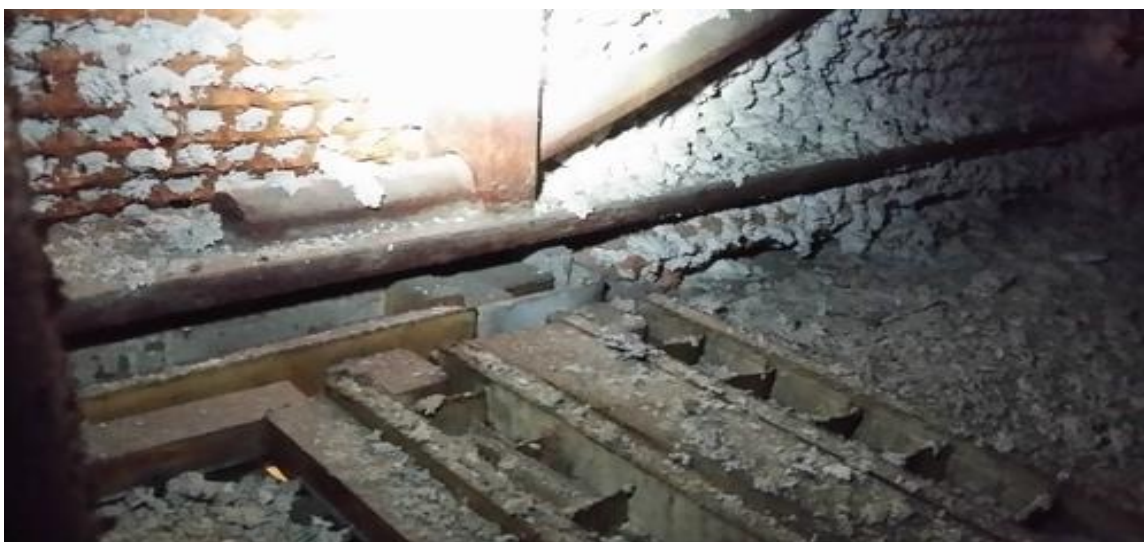
Sprayed asbestos on a column of system built school – Steel frame, wrapped in perforated steel with blown asbestos (note pattern on top left)
