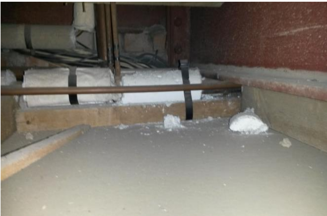
AIB debris in ceiling void of a school - insulation debris to back of non-asbestos suspended ceiling
