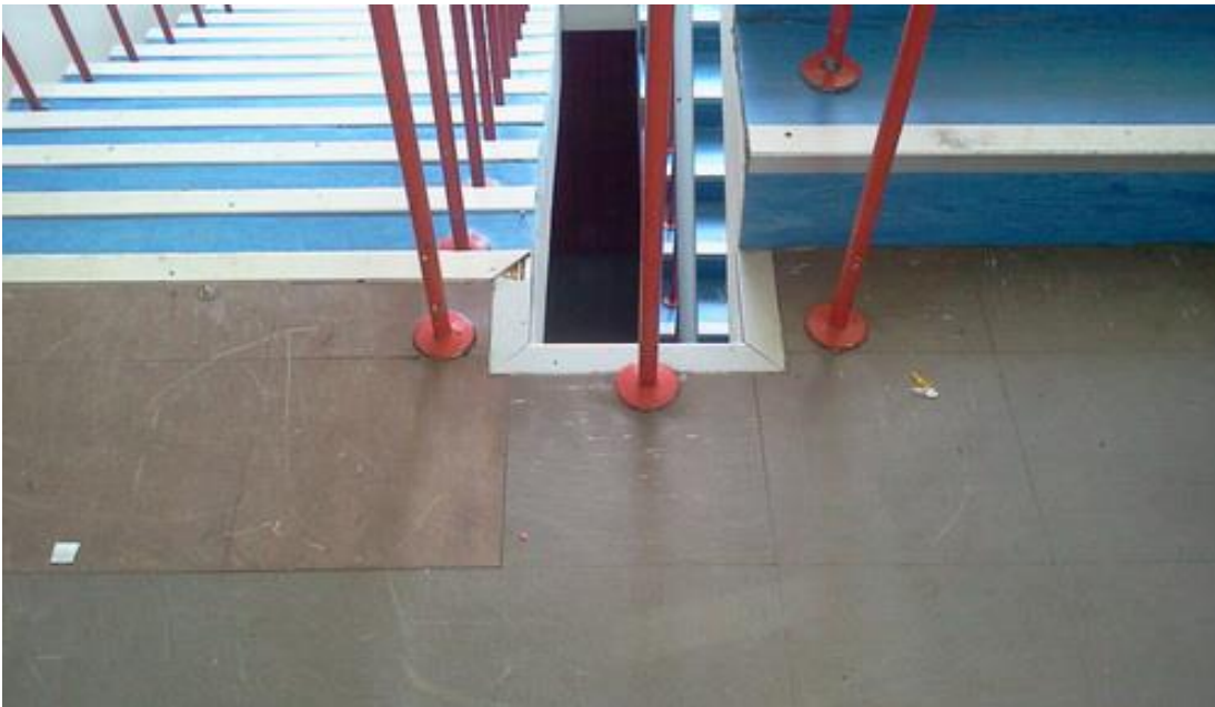
Asbestos containing stair nosing
