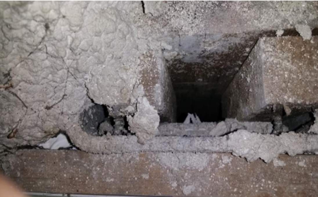
Sprayed asbestos on a column of system built school – lining behind cement wall end and column linings
