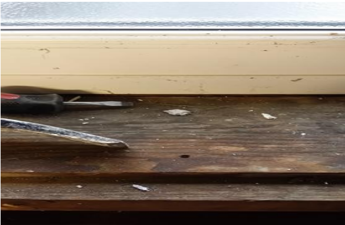
AIB cladding and asbestos debris – asbestos debris from AIB window surround cladding
