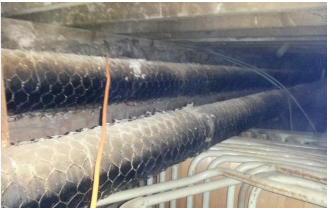
Asbestos lagging beneath floorboards
