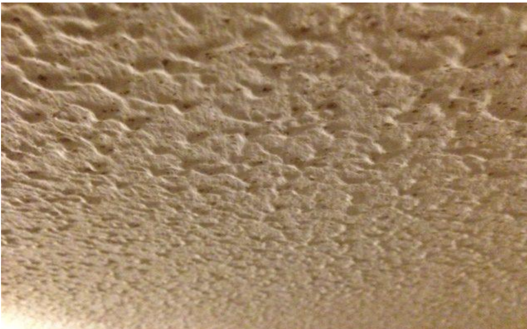
Sprayed asbestos on the ceiling of a school corridor – sprayed asbestos above suspended ceiling
