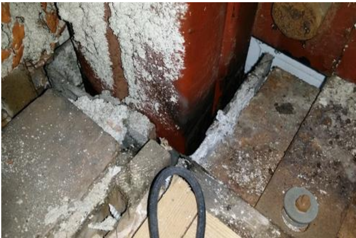
Base of a structural steel column in a classroom – exposed asbestos column linings
