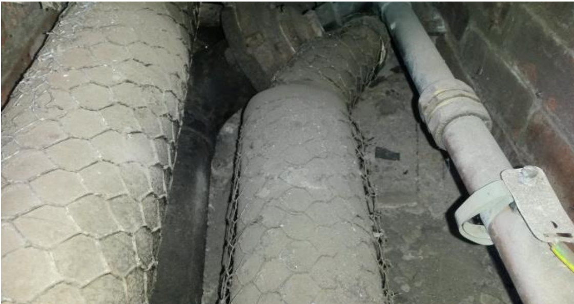
Asbestos in underground duct work- sub floor heating ducts, asbestos pipe insulation
