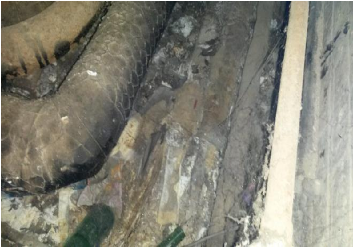
Dust containing asbestos - asbestos 'dust' pipe insulation below stage
