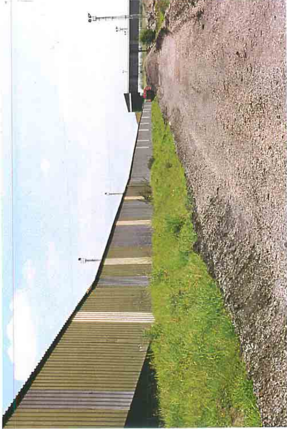
Char 1 & 2 Conveyors Showing a typical clad conveyor design
