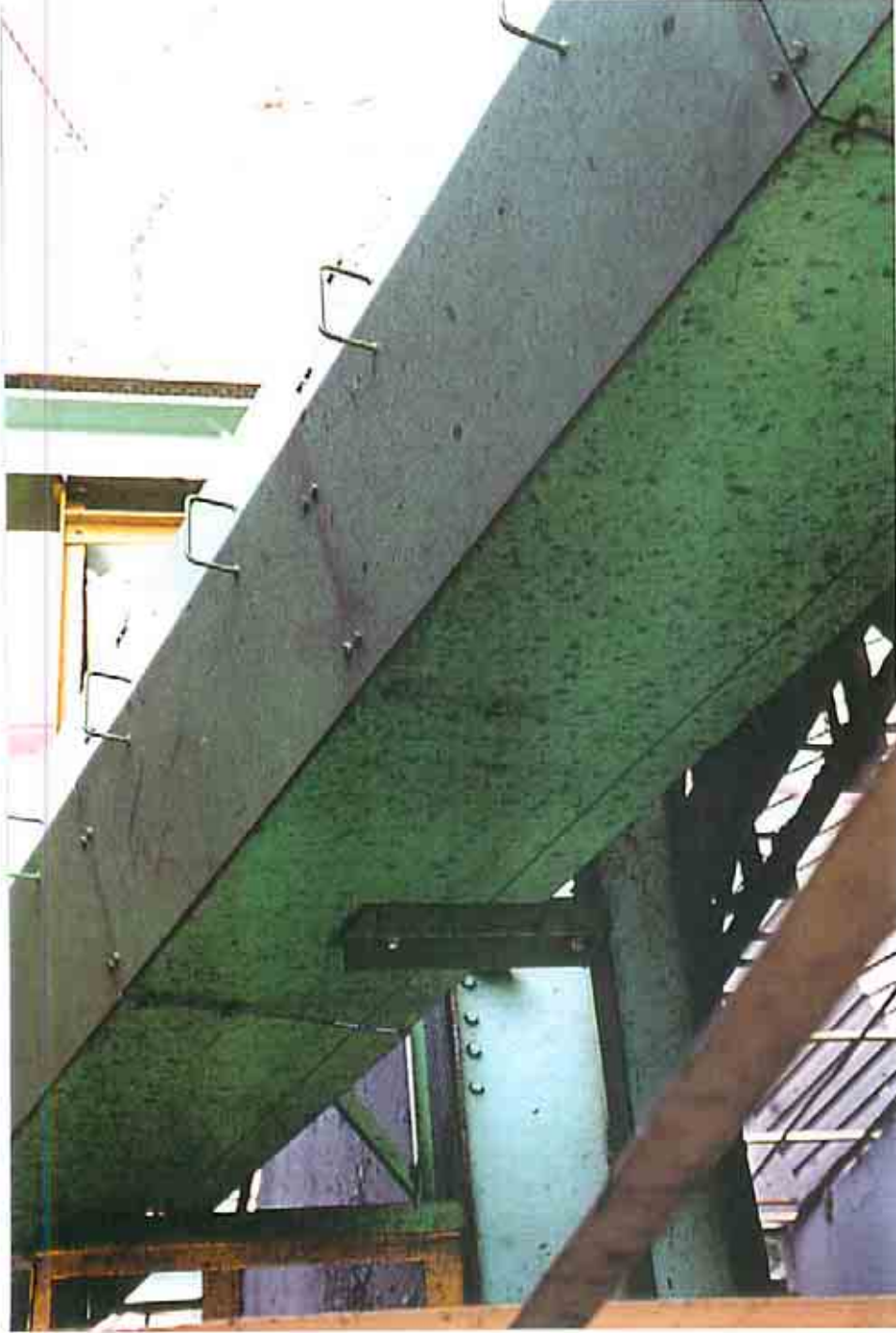
JD103B Conveyor Showing rubber conveyor enclosed by metal structure
